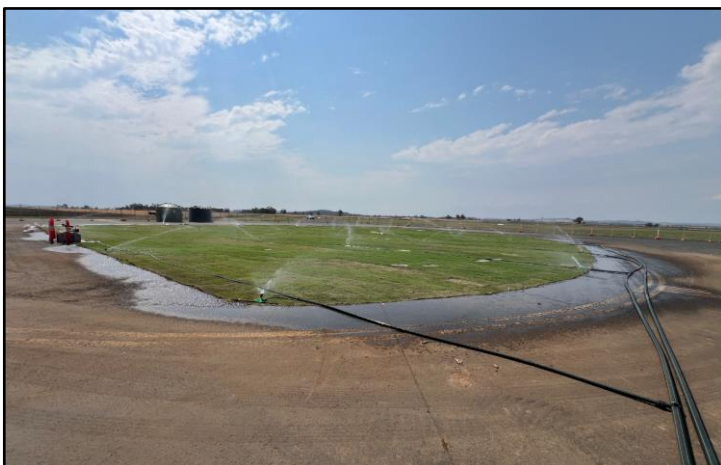
Remediated grass following soil excavation and stabilisation at the hot refuel area.
