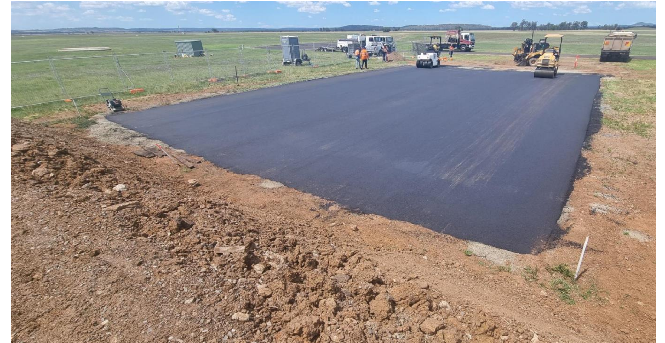
Delivery of asphalt at the Former Fuel Compound following excavation to support capping, November 2025.
