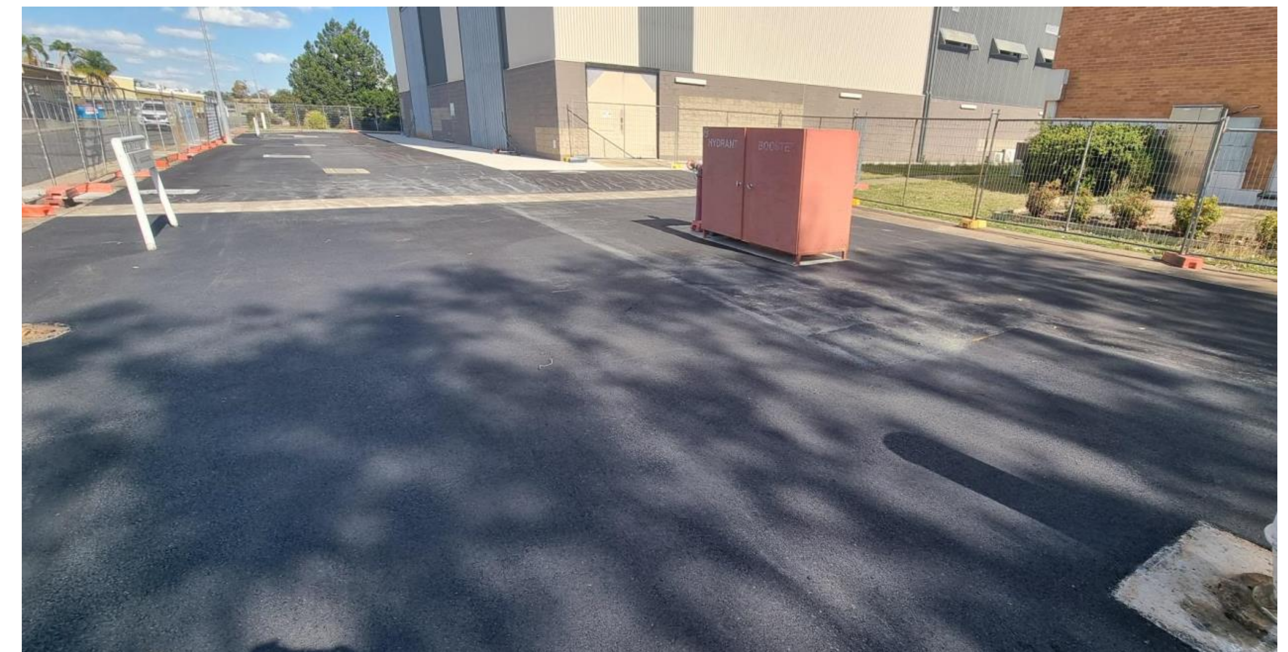
Delivery of asphalt at the Former Fire Station following excavation to support capping, November 2025.
