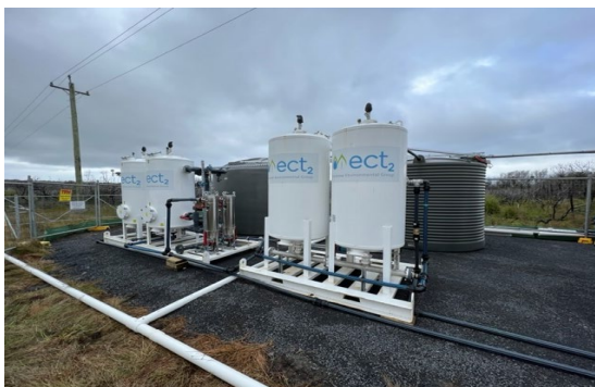
Interim water treatment plant at Jervis Bay Range Facility
