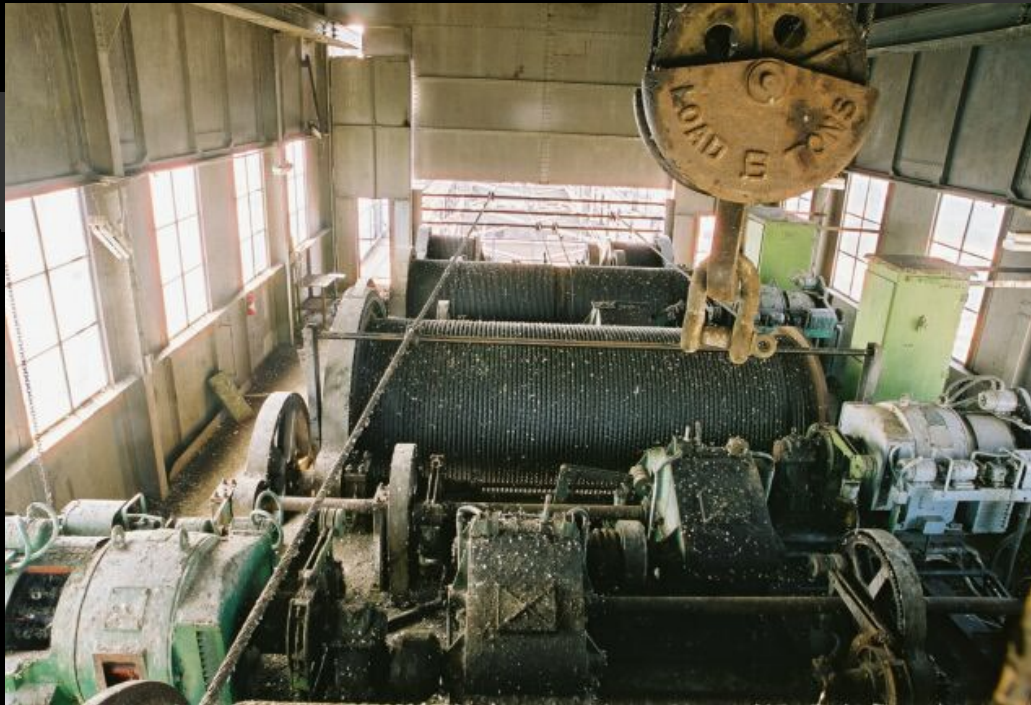
Main Motor Room
