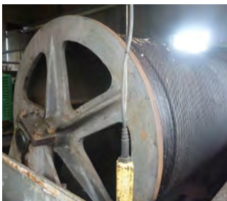
Hoist Drum Set (Source: GML)
