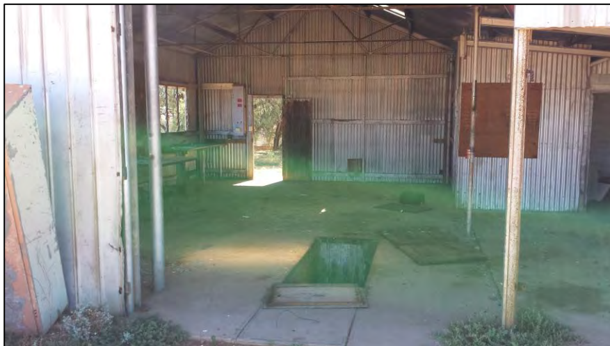
Plate 9: Vehicle service pit inside workshop near Main Homestead
