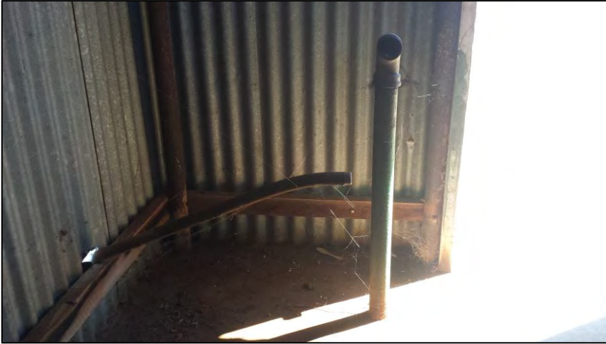
Plate 5: Fuel transmission line to inside of oil and fuel storage shed
