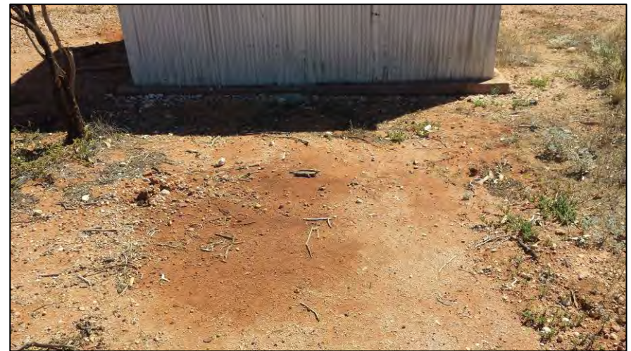
Plate 8: Surface staining at rear of oil and fuel storage shed beneath location of former diesel AST
