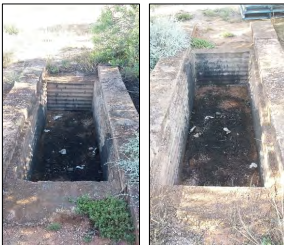
Plate 7A and 7B: View inside vehicle service pit adjacent to oil and fuel storage shed (staining in base)
