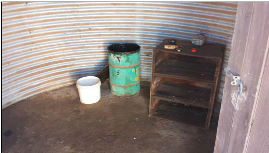
Plate 5: View inside oil and fuel storage shed; staining on concrete floor
