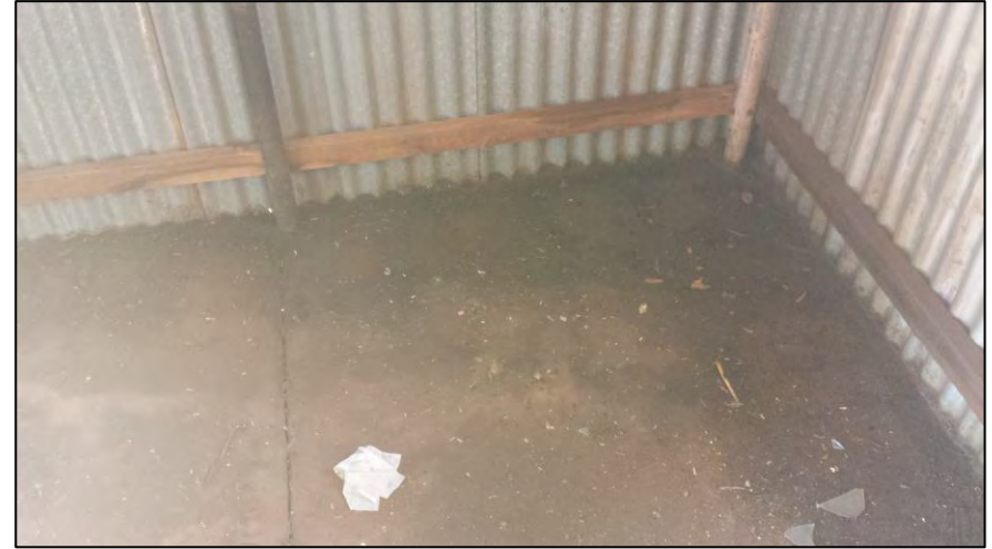
Plate 6: Staining on concrete floor of oil and fuel storage shed
