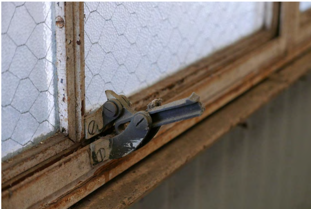
Plate 15 Hangar 257 – Close up broken latch – image 10513
