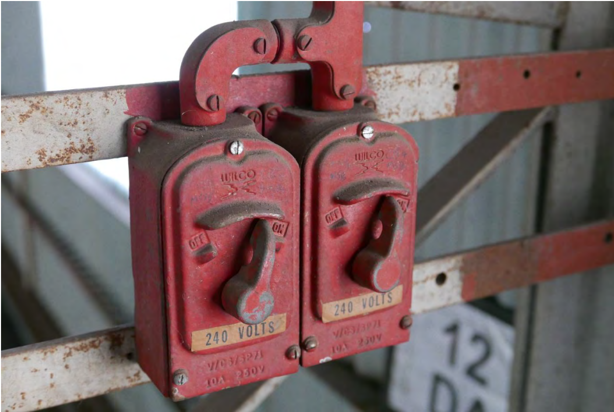
Plate 17 Hangar 261 – red WW2 period electrical switches – image 10659
