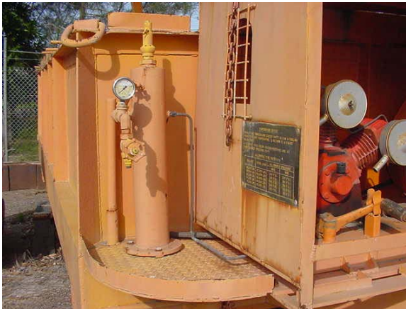
Side view of compressor compartment
