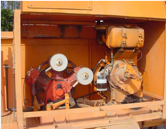
Close-up view of diesel compressor
