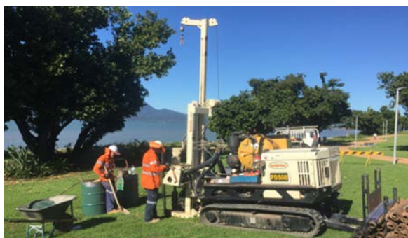
Example of a typical drill rig used to bore holes for sampling.
